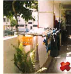
Installation of fixed laundry rack at common corridor. 衣架固定安装在公用走廊。
