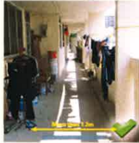
Clear width of 1.2m with placement of foldable/removable clothing rack. 置放可折叠/移除衣架后,走廊的净宽度为1.2米。
